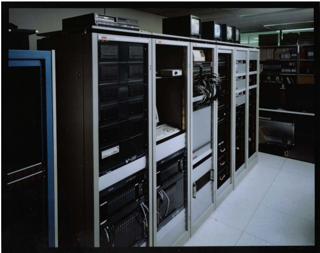
Video Server Room – Equipment Supplied by AWA
